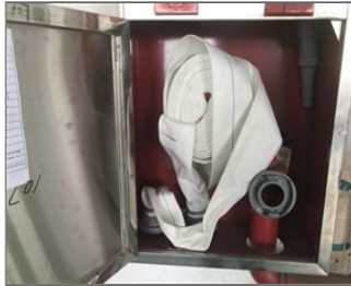
Photo of fire safety equipment 42 Fire hydrant.JPG
