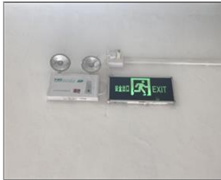
Photo of fire safety equipment 44 Exit sign and Emergency light.JPG
