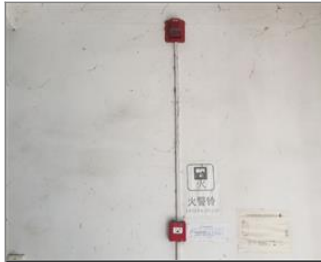
Photo of fire safety equipment 43 Fire alarm.JPG
