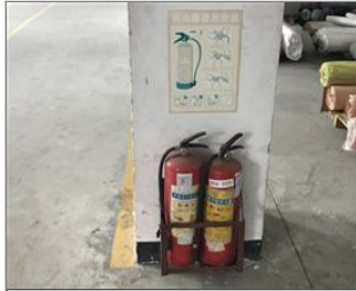
Photo of fire safety equipment 41 Fire extinguishers.JPG
